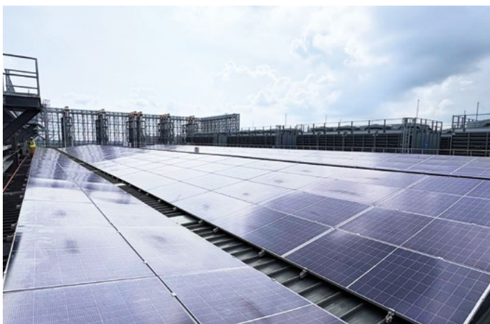
Powering sustainable operations with renewable energy at DC Tuas
