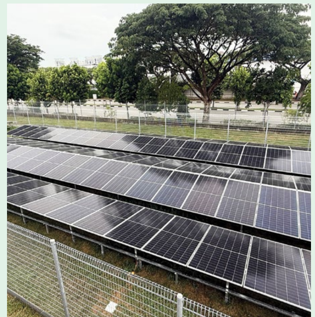
Solar PV installation at NCS Bedok
