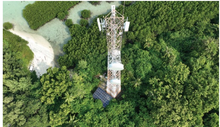
Solar-powered base station
