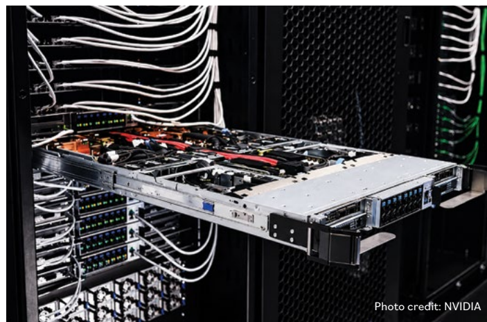
Next-generation GB200 cluster deployment with direct-to-chip liquid cooling
