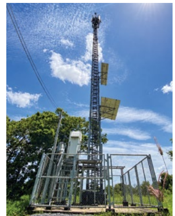
Solar-powered base station
