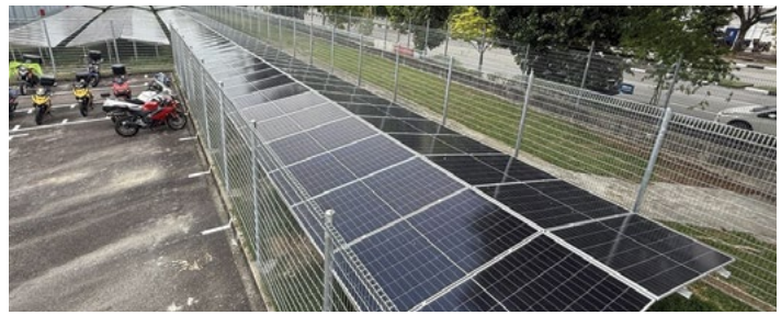
Newly installed solar PV systems at NCS Bedok
