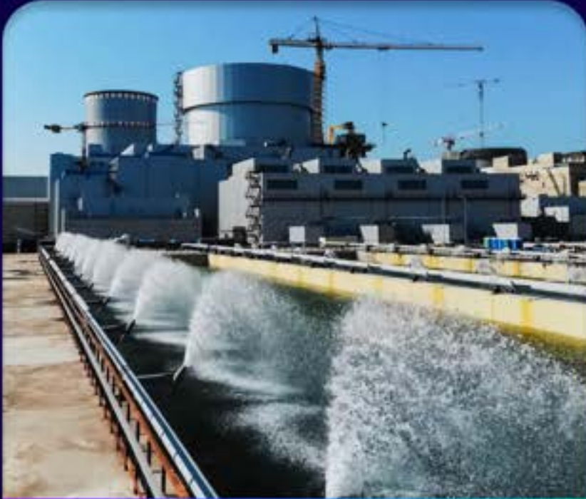
Recycled water for cooling systems
