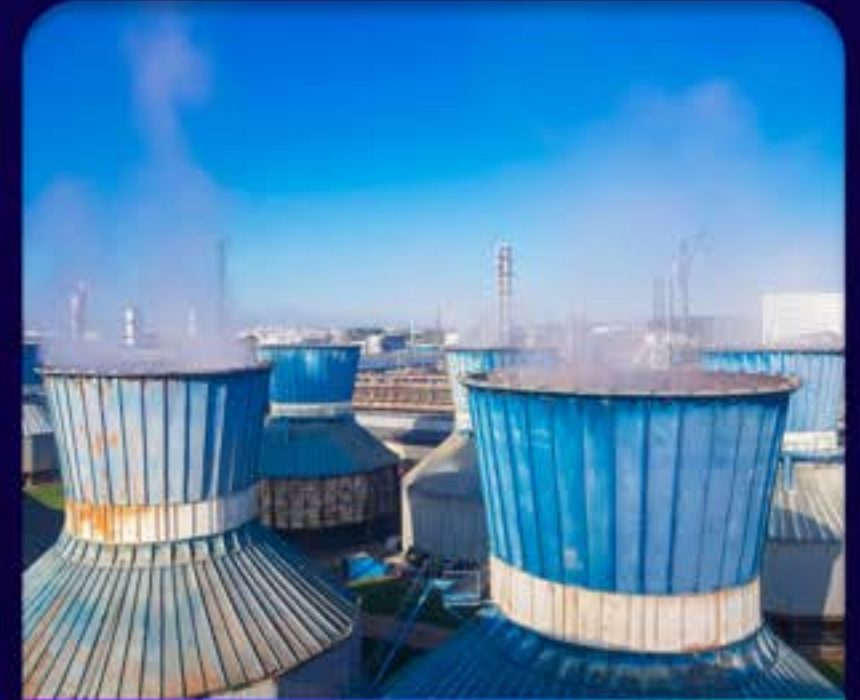
Cooling tower blowdown reuse
